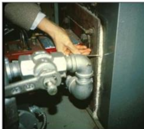
Rope gasket at boiler plate
