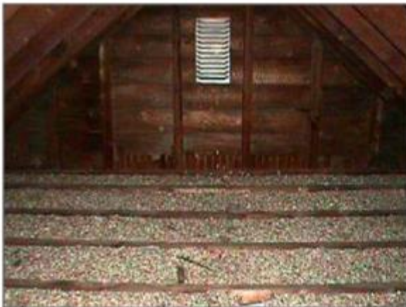
Vermiculite attic insulation
