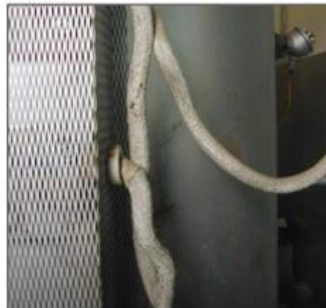
High Voltage cable insulation
