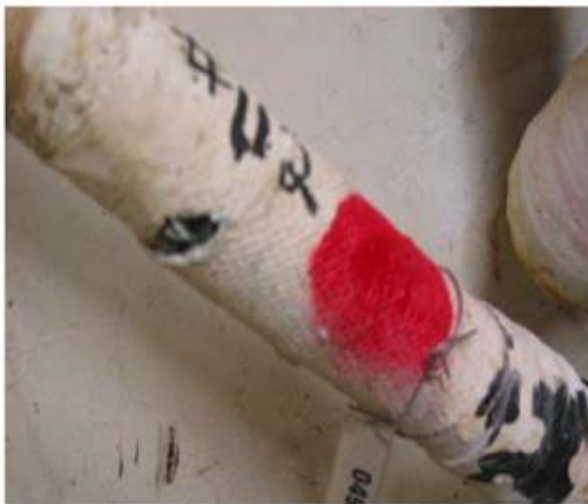
Asbestos Pipe Marking
