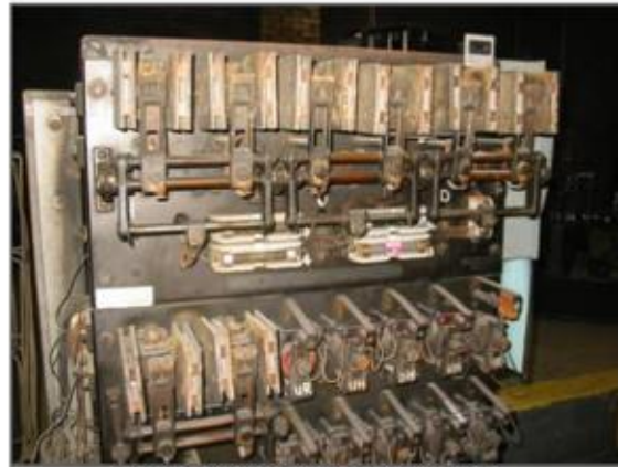
Transite Blocks in Elevator Switchgear
