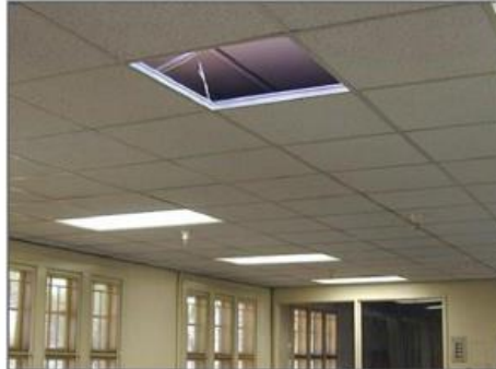
Lay-in ceiling tile
